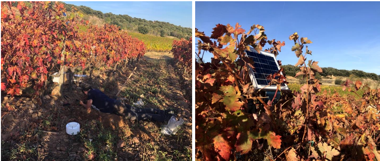
Figure 4. Installation of soil humidity sensors and final solar panel in the old-term vineyard in Tudelilla site (Vivanco winery), La Rioja.
